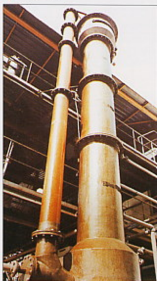
Colonne pulsée industrielle. Industrial pulsed column.
